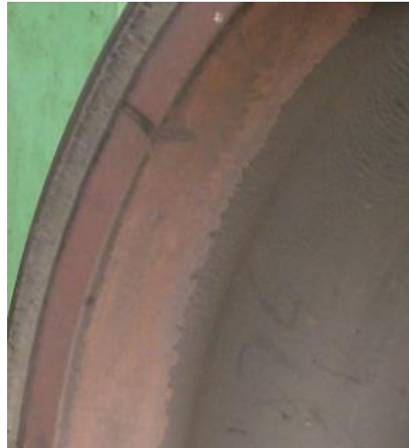
Old and fresh burnt paint
